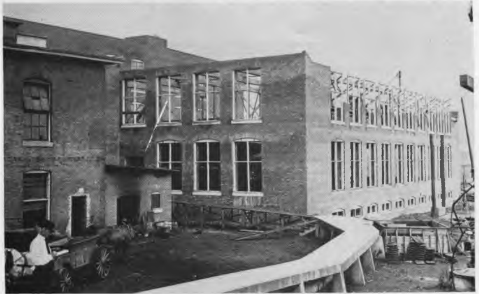
This photograph was made on July 17, 1920 while No. 1 "Kitchen" was under construction. At that time the cotton conveyor pipe ran from the opening room beneath a concrete walkway to No. 1 picker room. Cartload of dirt or gravel are visible at the left. Work on the building appears to have reached the second story. (Photograph Property of Huntsville Mfg. Co.)
