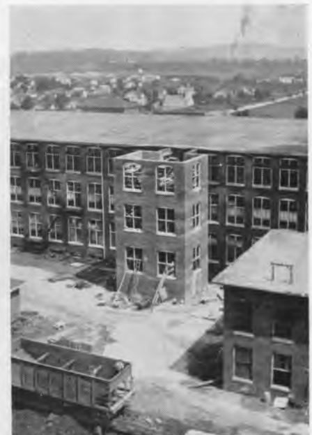
This picture was made on July 24, 1920. At that time the extension to No. 1 mill was under construction at the east end of the mill and the toilet towers which had been at the east end were torn down and new toilets built on the south side of the building. Toilet towers on No. 2 mill were not changed after the original building was finished.
