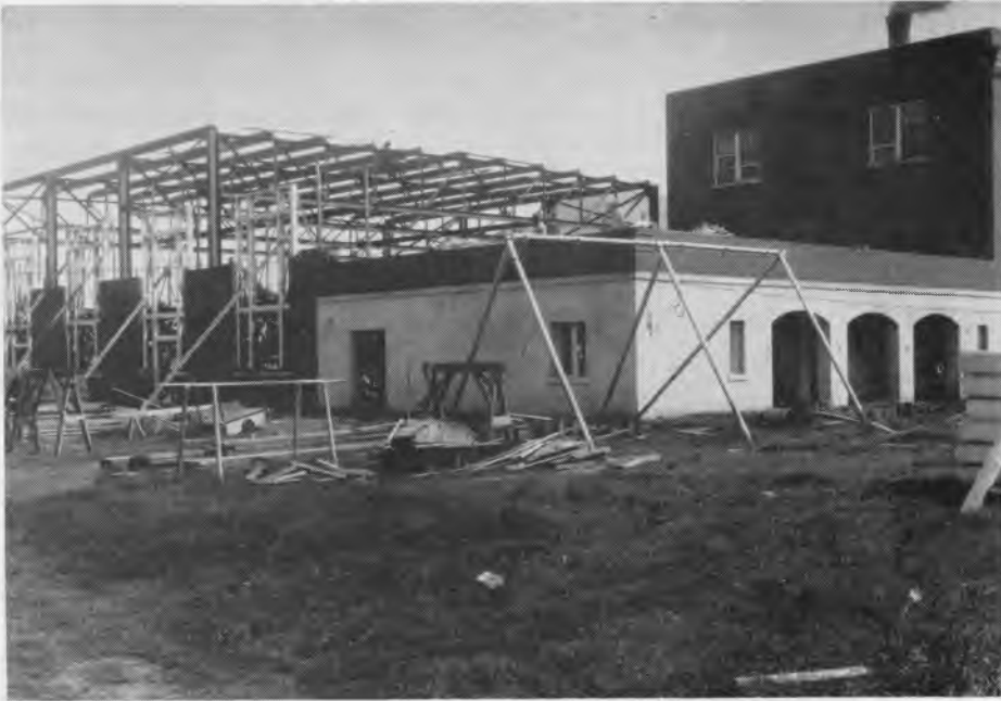
This view shows the construction of the school auditorium and additional rooms in 1928. Expansion of Joe Bradley School was undertaken several times by Merrimack Mfg Co., after they built the first section in 1919.
