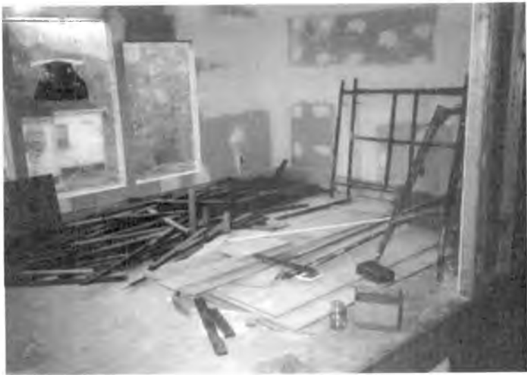
Looking out through the new window openings that are covered with plastic. The wood is some of the flooring my sister, Gail, salvaged from a building in Oak Ridge, Tennessee.
