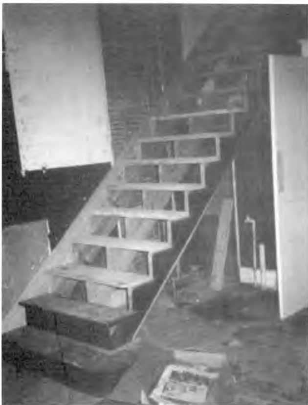
The staircase, taken from the EastBrook Springs Resort, during installation in the kitchen.
