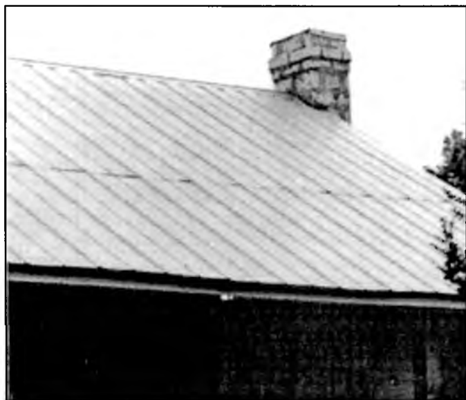
Fig. 10 Chimney detail, yeoman's house, Oran Whitaker Road between Nebo and New Hope-Cedar Point Roads, Madison County. Courtesy Debra Miller.
