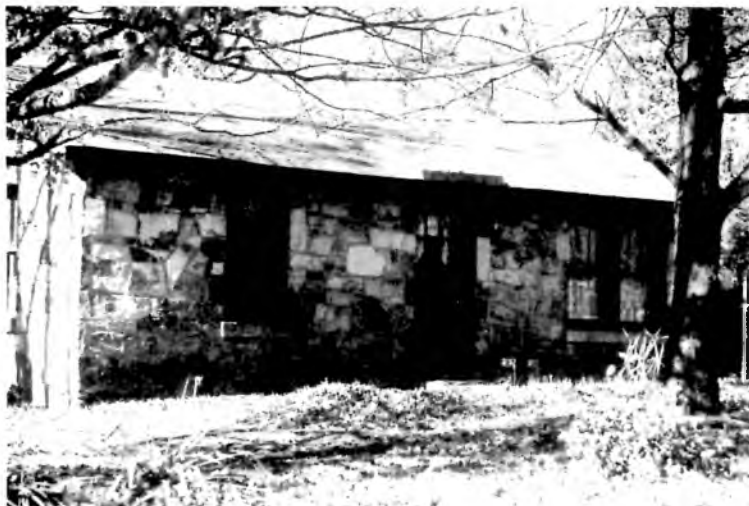
3618 Fearn—Random range rubblework on a solid stone wall home. The stone window sills are sloped away from the window and contain a drip edge (a shallow groove underneath the front edge) so that water drips to the ground instead of running back toward the stone where it can wear away mortar. Photo by H. Cross.
