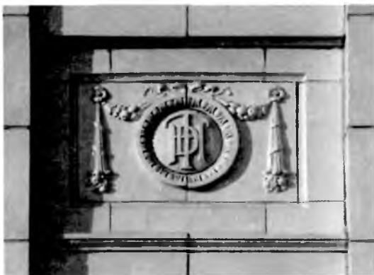
One of the terra cotta panels used to separate the windows between floors. This design was used on the two-story base; HDT, for Huntsville Daily Times, is encircled and bedecked with rippling ribbons and swags of fruit and flowers. Photograph by Scott McLain
