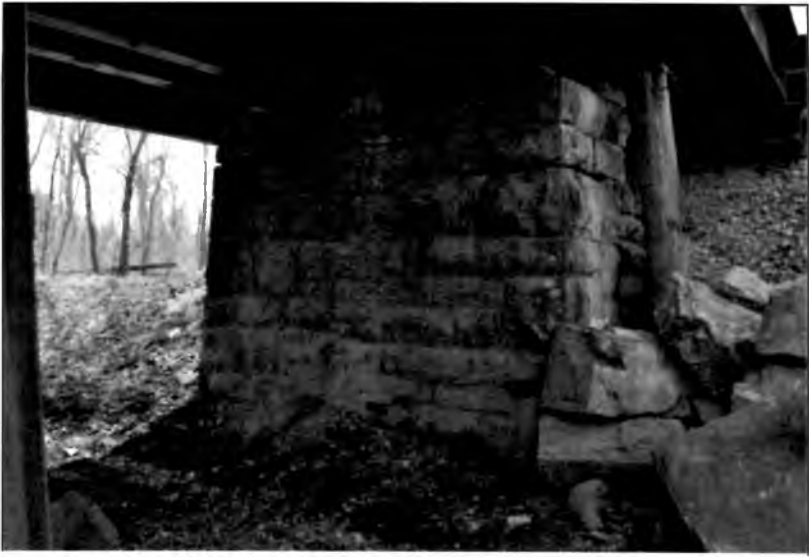
Original pier of the Memphis & Charleston Railroad Bridge across Indian Creek; a pier still stands on either side of the creek, even though neither is used for support anymore.
