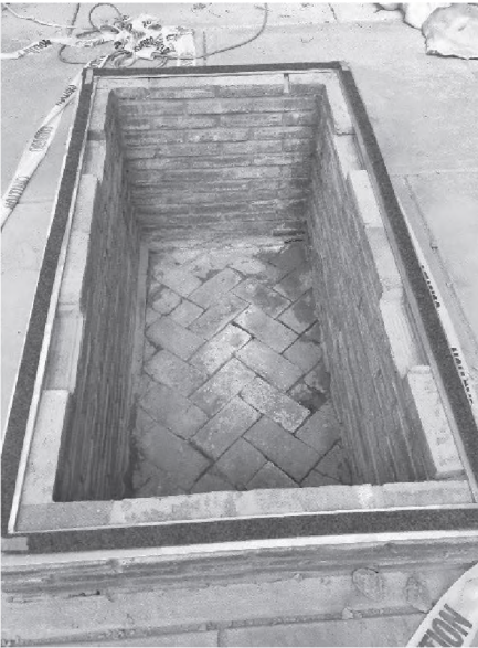
The old sidewalk's herringbone pattern emerges during construction of its new aluminum frame.
