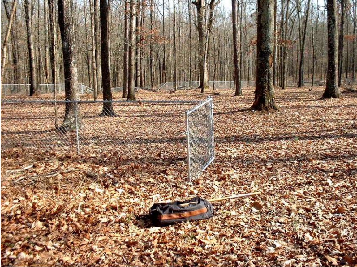
Green Grove Cemetery, Redstone Arsenal, Madison Co. AL., March 11, 2003 Entrance gate, fence damage in background
